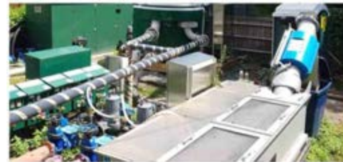
Photo of groundwater treatment unit.
